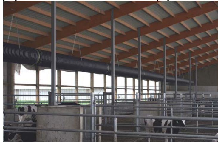
Figure 8. The air distribution duct in this barn is a firm “flume” pipe usually used for drainage and other heavy duty purposes. It can withstand wind in relatively open situations.
