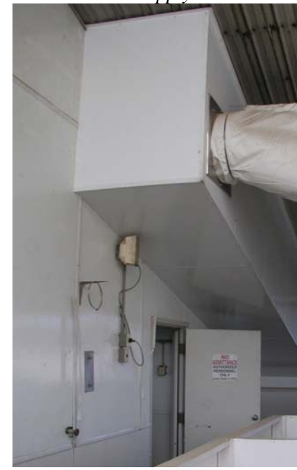
Figure 3. Because of a utility room on the left, a passive air supply duct was constructed to side wall. The fan and tube were mounted in the supply duct.
