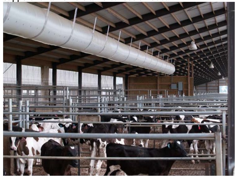
Figure 6. Plastic freezer strips used to provide additional support for a flexible air distribution duct.
