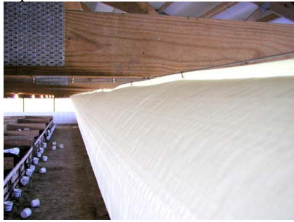
Figure 5. The support cable runs the length of the barn and is supported by the building ties. The tube is attached to cable with clips.
