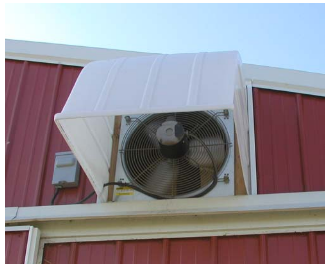
Figure 2. A fan and hood that are very close to the roofline and which sometimes catches snow as it drifts off the roof and propels it into the tube inside the barn.
