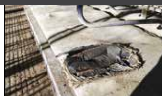
A damaged mattress prior to repair
