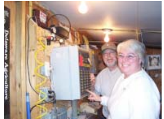
Diann and Brian McCahill at the controls of their water pressure adjustment system.
